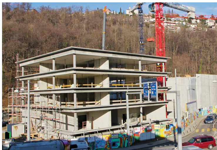
The new building in Lugano with on the left side the administrative building and on the right the machine room.
