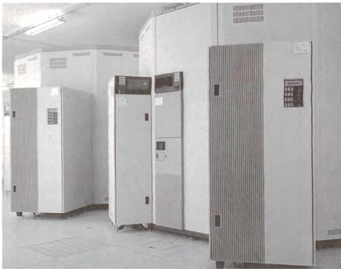
Storage Tek silos for archiving of large amounts of data.
